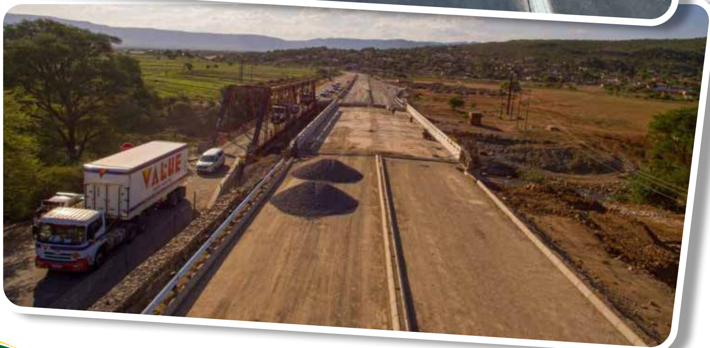
Visible progress is being made at the new bridge in the Sekhukhune district
